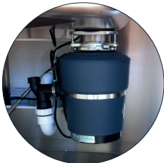
Waste disposal unit
